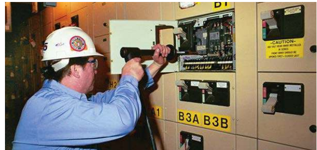
MCCB testing using the HCP2000
