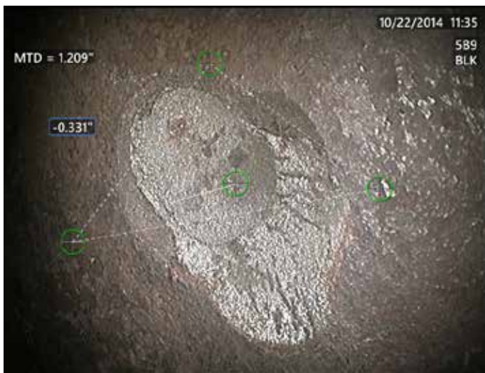
Surface Pit Normal View with Depth
